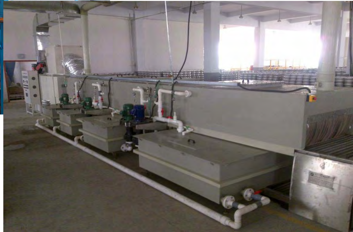
Automatic Washing Line
